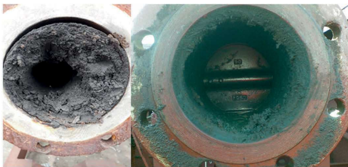
Fig. 1. Example of a pipeline that is blocked due to the deposition of paraffin on the walls 9)
