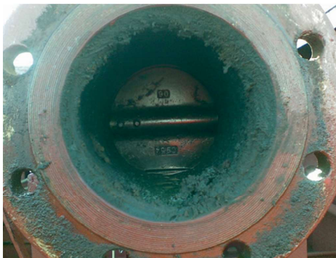
Fig. 1. An example of a pipeline blocked due to paraffin deposition on the walls 5)
